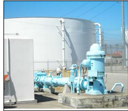
Photo 1 – Water well and storage tank
