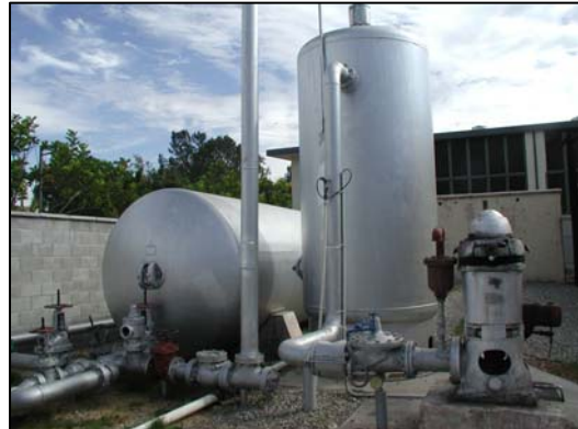
Photo 2 – Small water system well and storage
