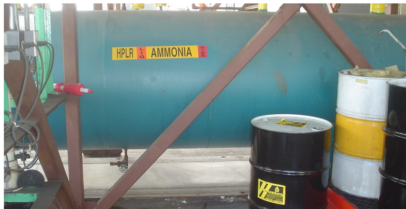
Ammonia refrigeration vessel with refrigeration oil storage
