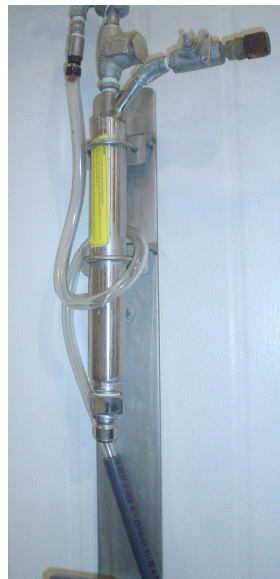
Wash Station with chemical feed
