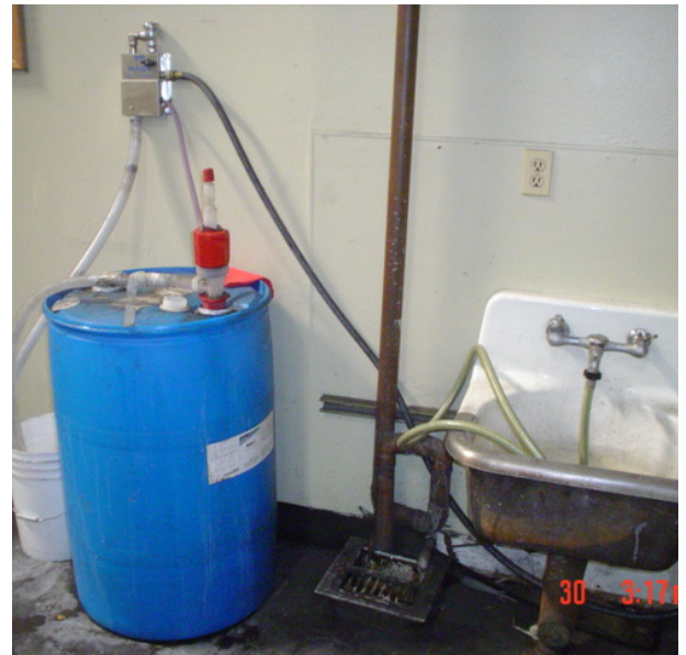
Chemical Mixing Unit
